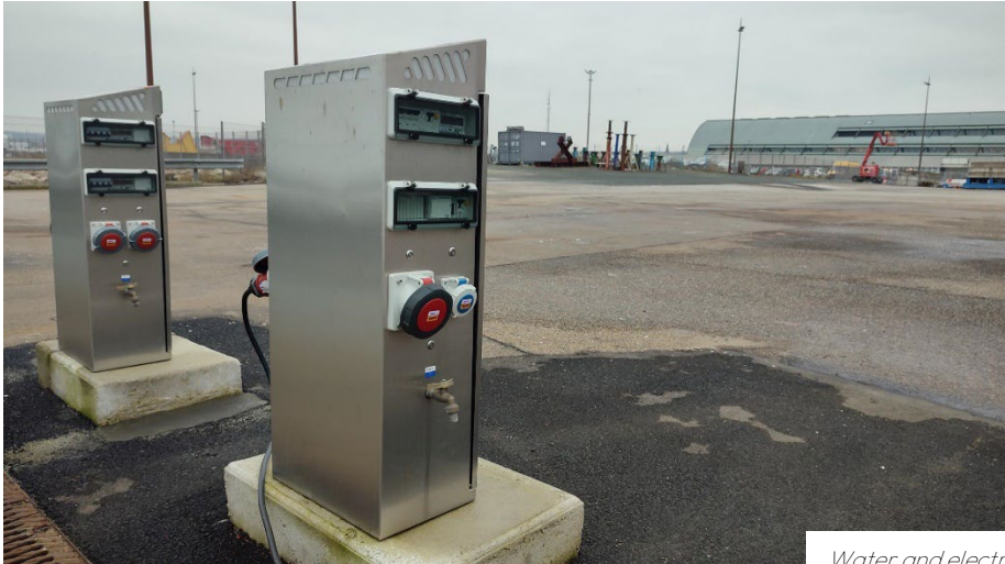
Water and electricity station @PortsdeNormandie
